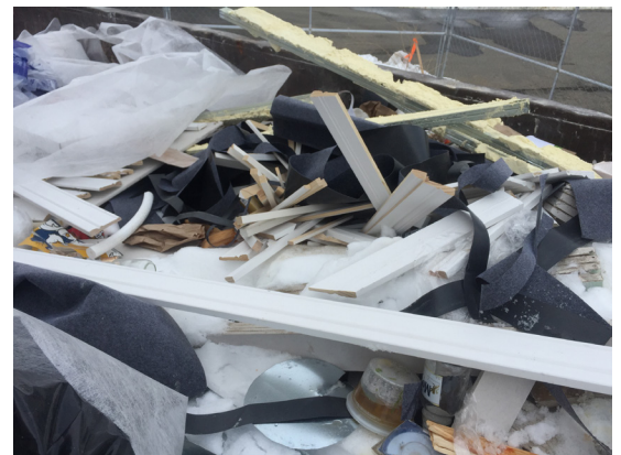
Materials collected in a mixed container were sent to a C&D sorting facility.
